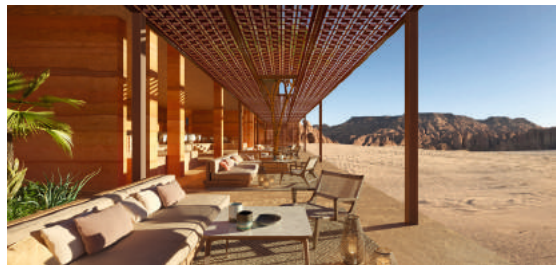
Ashar Tented Resort (Accor - Banyan Tree) in AlUla, Kingdom of Saudi Arabia designed by AW2 Architecture Workshop led by Reda Amalou and Stéphanie Ledoux. Under construction.
